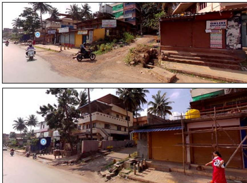
Fig 16: Broken footpaths and drainage clogging need to clear for pedestrian movement.
