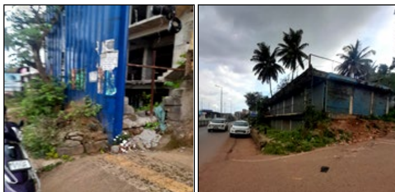
Fig 17: Issues with old and unused buildings along the footpath and under constructed buildings with GI sheets barricades falling on footpath.
