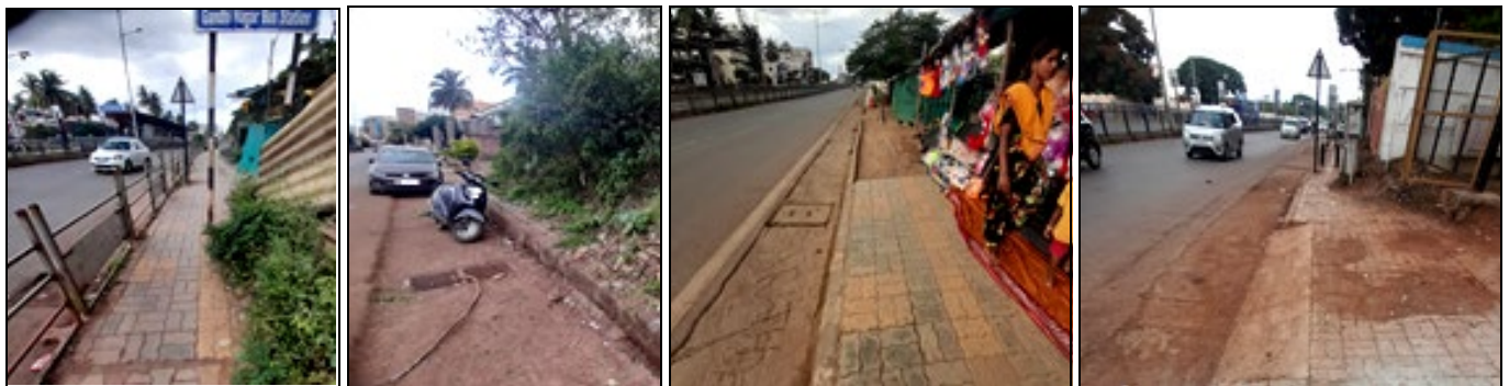
Fig 13: Encroachment of footpaths on both sides of the road
