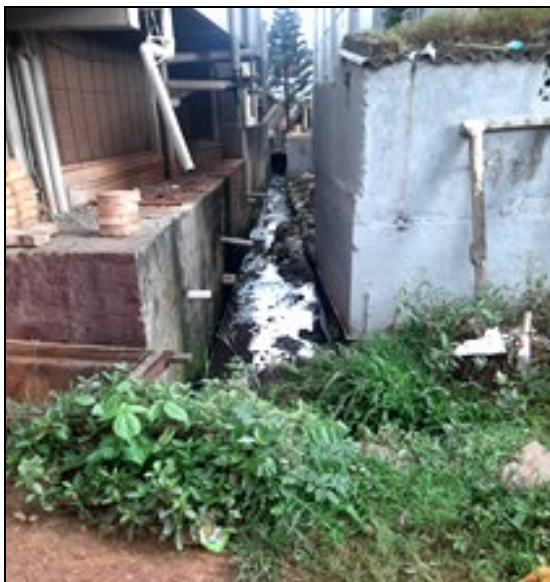
Fig 20: Pond overflows during the rainy season due to the breakage of pond bund long ago, this is due to the loose soil. All overflow water flows through narrow naala inside the YS colony area. Which overflows in residential areas and blocks the easy flow of other drainages.
