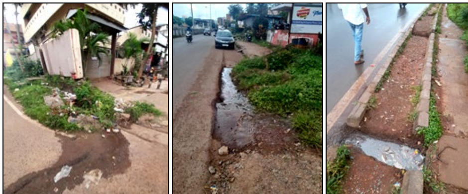
Fig 15: Drainage overflow from hilly regions of Vidyagiri and Gandhinagar area onto the main road, blocks pedestrian movement.
